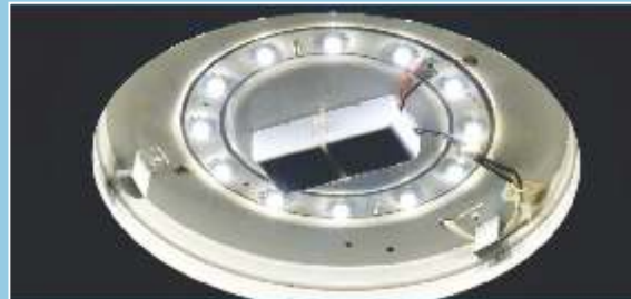
LED Lights at the Orchid Crown site
