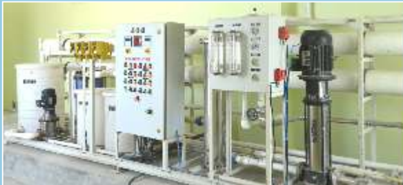
RO Plant at CTS Siruseri
