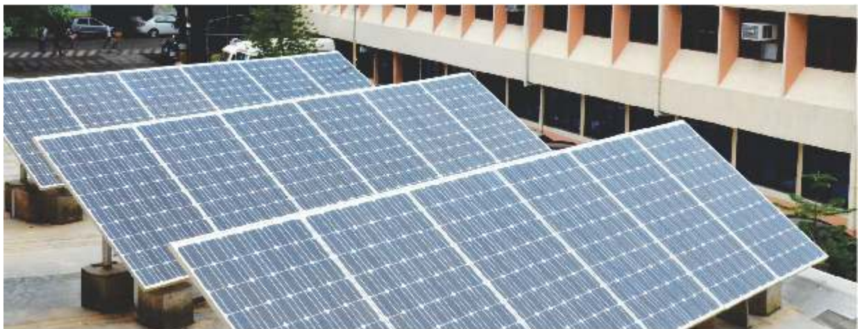
Solar PV panels installed at Powai campus
