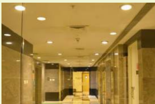
LED lighting at L&T's Campuses have helped reduce energy consumption
